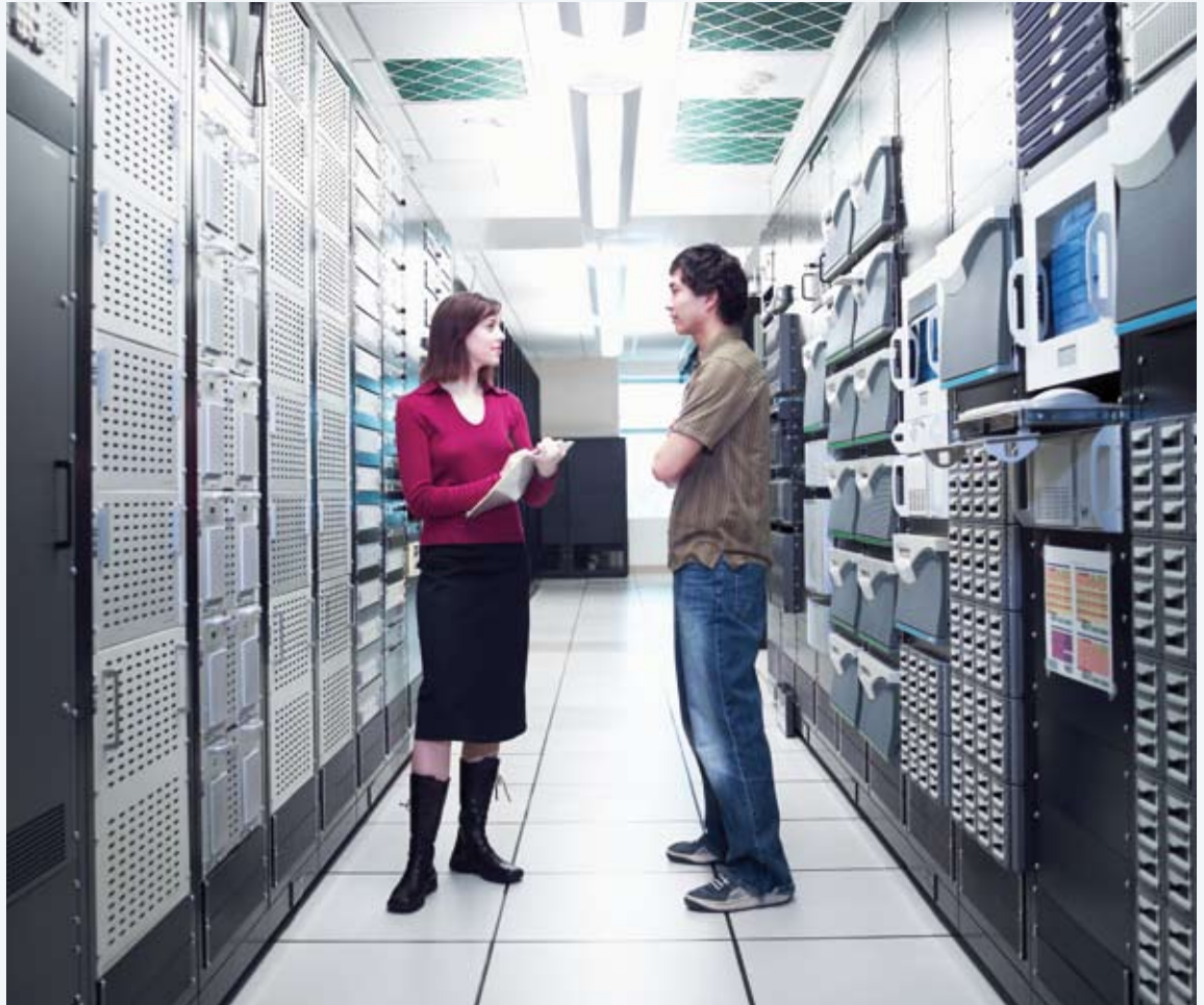
Chloride provides technology to protect data centre power supplies, ensuring that company systems continue to run smoothly.
